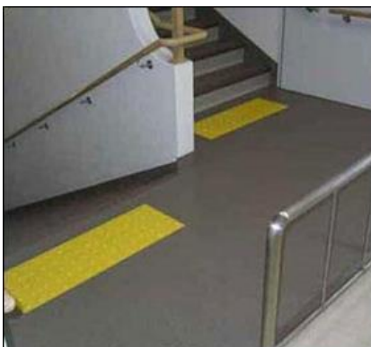
Figure 7-9: Warning blocks at landings
